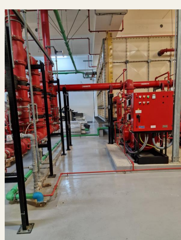
Typical firefighting system installations
